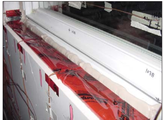
Figure 8. Sealing the window frame to the air barrier at the interior side
