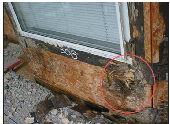
Figure 1. Damage caused by water entry
