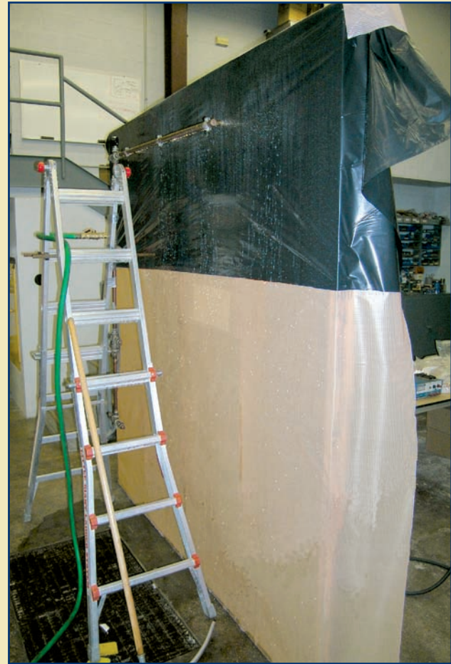
Figure 8. Modified spray test setup utilizing reduced water spray onto a polyethylene sheet. Water runoff was allowed to wet the WRB for 30 minutes.
