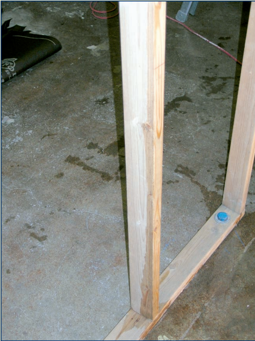
Figure 7. Water penetration is evident on the wood test frame after removal of the WRB at the completion of the 15-minute direct water spray test.
