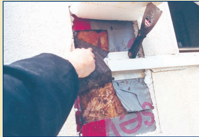
Figure 3. Example of exterior wall sheathing damage due to water penetration through a polymeric WRB.
