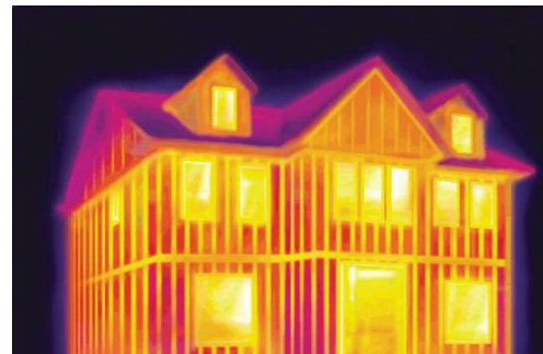
Thermal imaging illustration of unmitigated framing thermal bridges releasing heating energy (no continuous insulation).
