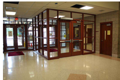
School security vestibule in addition to dual entry outer vestibule
